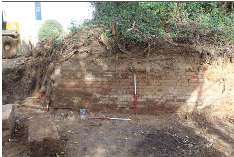
Plate 8. Northern and central sections of northern wall (51), looking North-east, with large "coping stones" in bottom left hand corner. Scales: 1m x 2.
