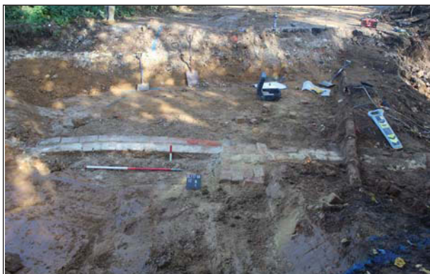
Plate 5. Northern section of southern wall (52), showing probable buttress. Scales: 1m and 0.20m.
