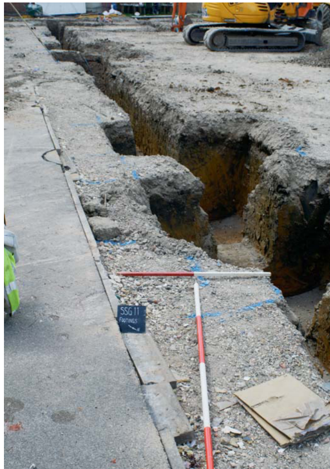
Plate 2. Footings in south-east area of the site, looking south-west, Scales: 1m and 2m.
