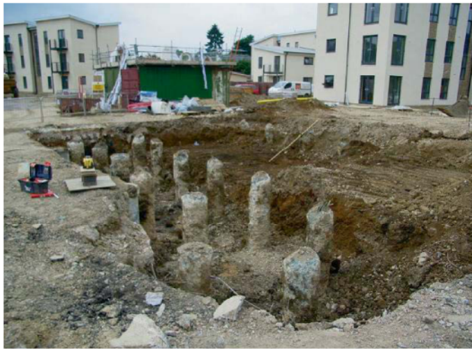
Plate 1. Bridge support area, looking north west, strip in progress uncovering piles in north.
