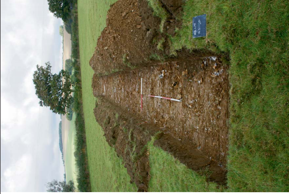
Plate 2. Trench 3, looking north west, horizontal scales: 2m and 1m, vertical scale: 0.5m.
