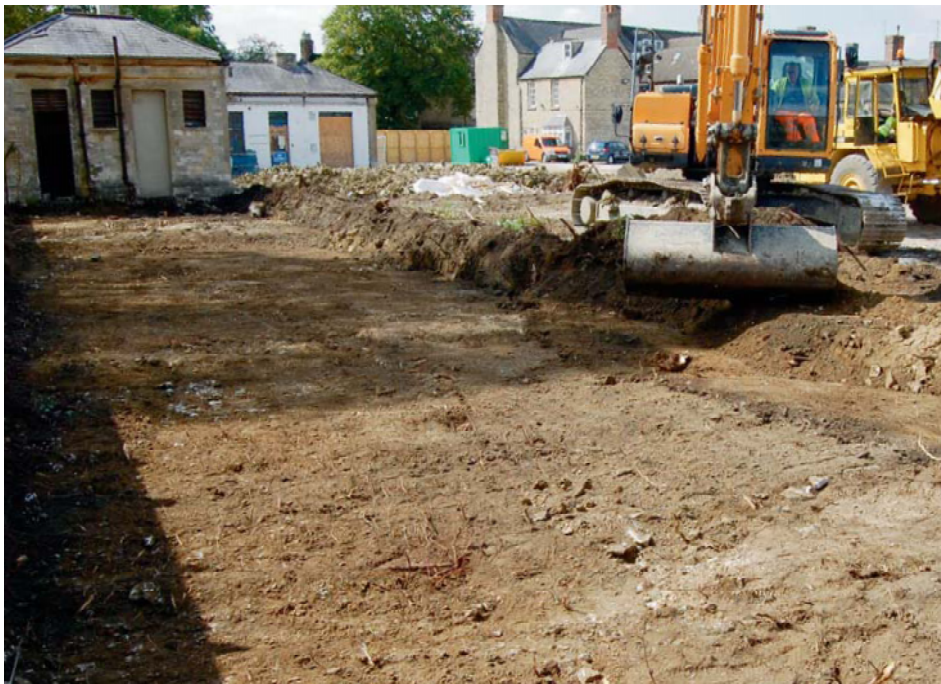
Plate 1. Watching brief strip for topsoil screening looking south east with station building in background.
