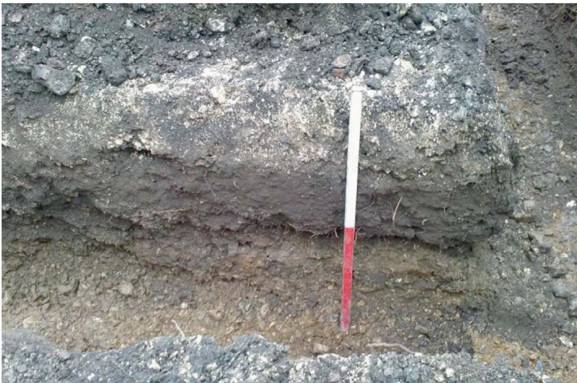
Plate 2. Footing trench, eastern end of central footing, looking south east, Scale: 1m.
