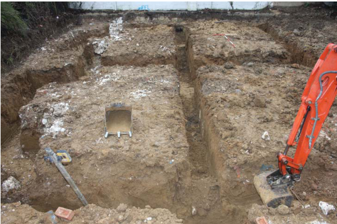
Plate 1. Footing excavation to south with wall 1 on left side of shot, looking south west.
