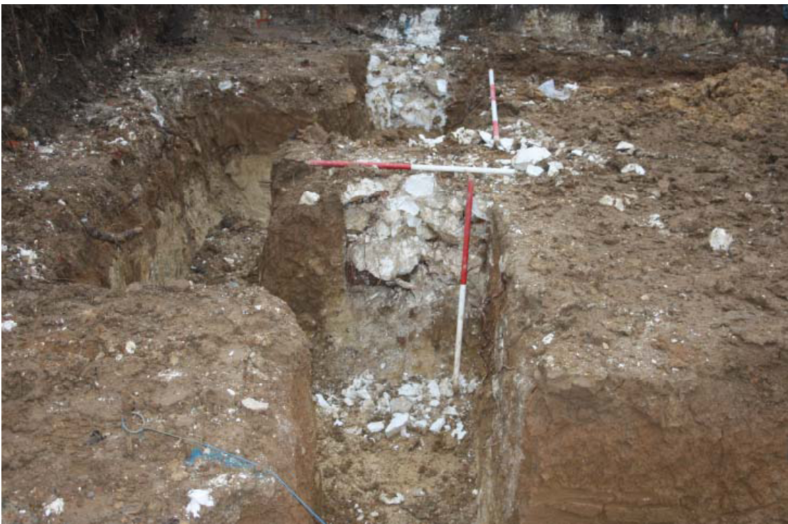
Plate 2. Wall 1 section in new southern footing, looking south west, Scales 1m and 2m.
