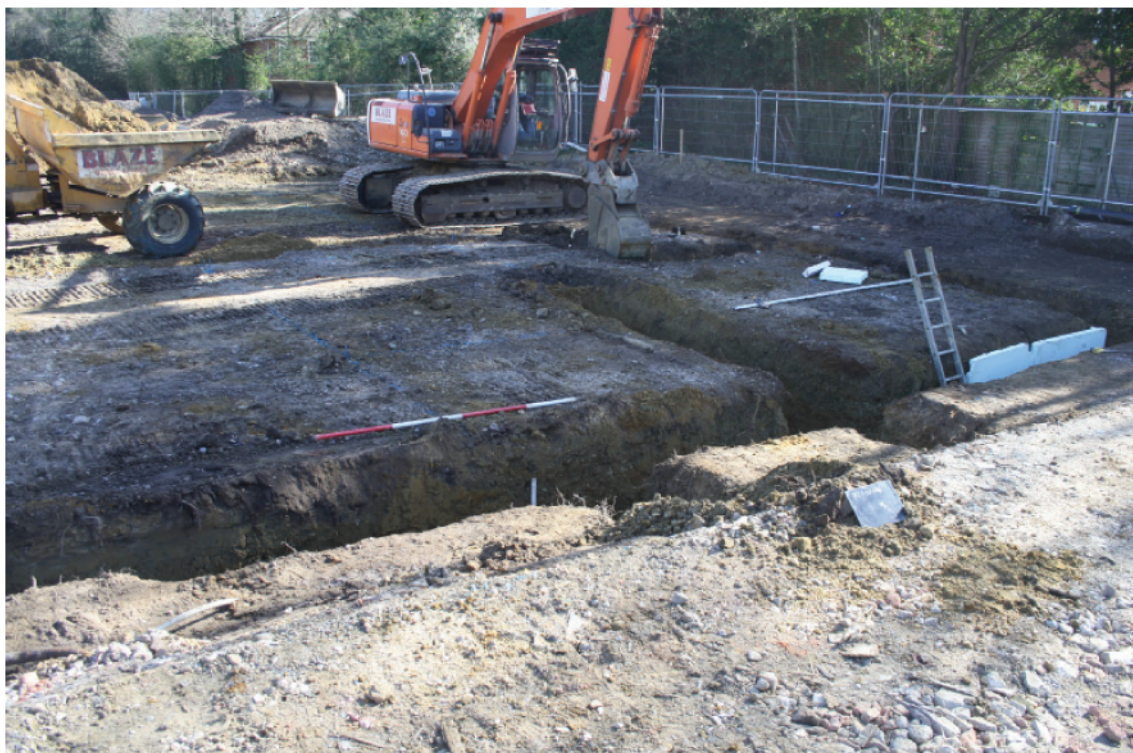
Plate 2. Excavating the footings for Plot C, looking northeast. Scales: 2m and 1m.
