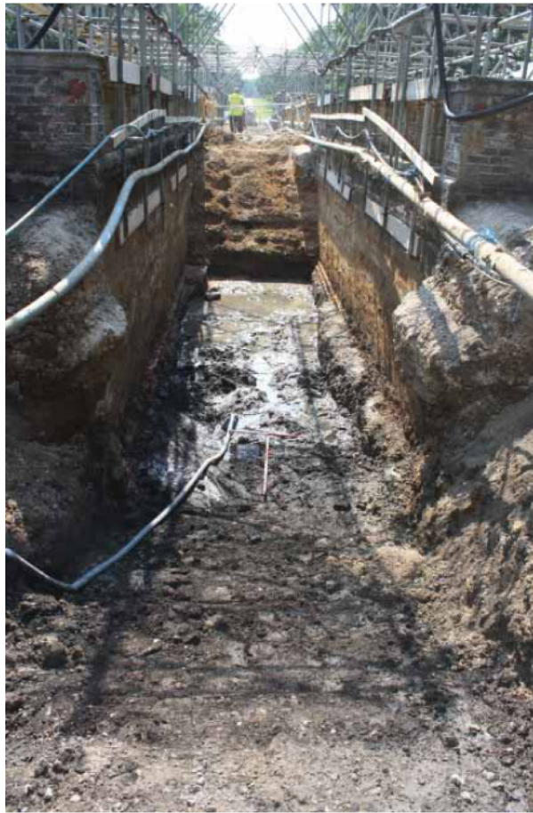
Plate 3. Deepest part of the interior bridge excavation, looking south west, Scales: 2m and 1m.
