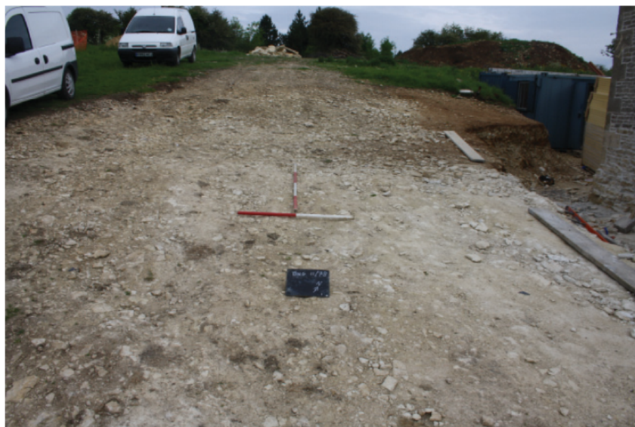
Plate 4. Exterior of barn showing area stripped of overburden with partially stripped area beyond. Looking north west, Scales 2m and 1m
