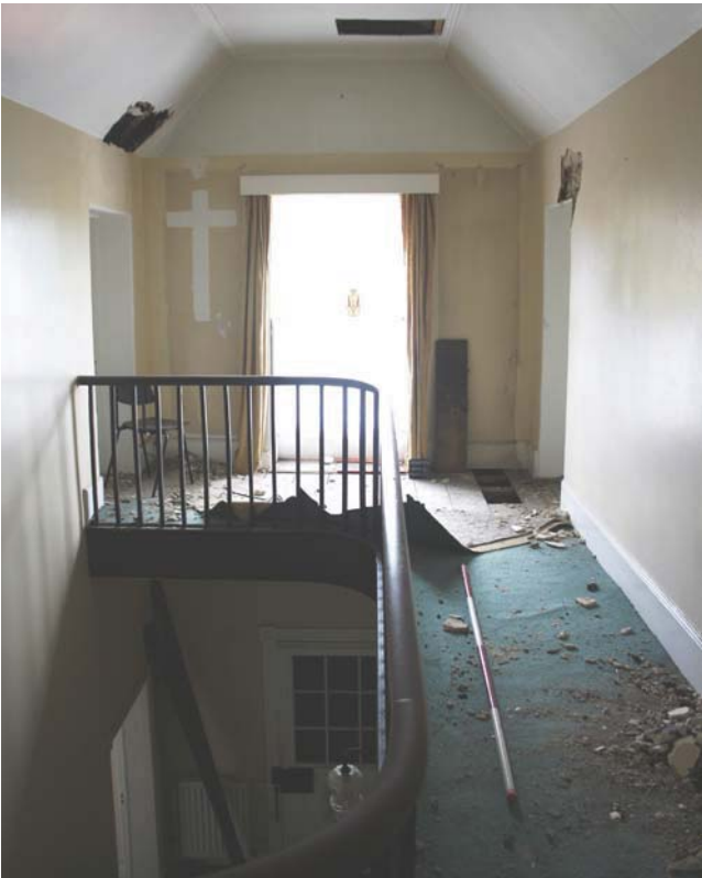
Plate 15. Room 26, view to window showing balustrade, looking south, Scales: 2m and 1m.
