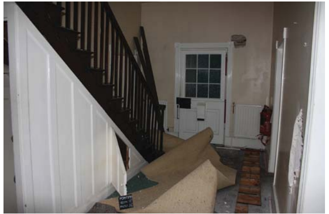
Plate 4. Room 12, view to door, showing stairs looking south east, Scales: 2m and 1m.
