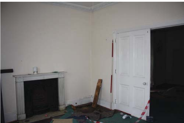
Plate 7. Room 3, view to double doors and fireplace, looking north west, Scales: 2m and 1m.
