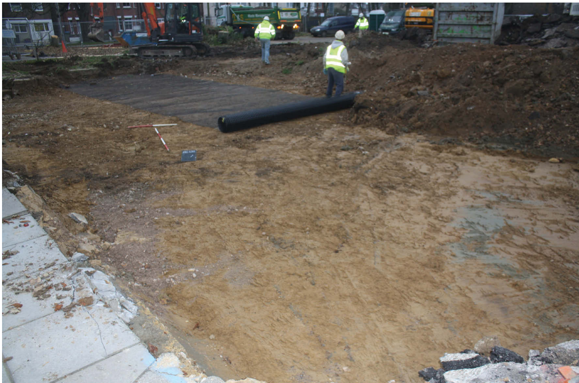
Plate 2. Exposed brickearth in process of being overlain by geotextile, looking north west, Scales: 2m and 1m.
