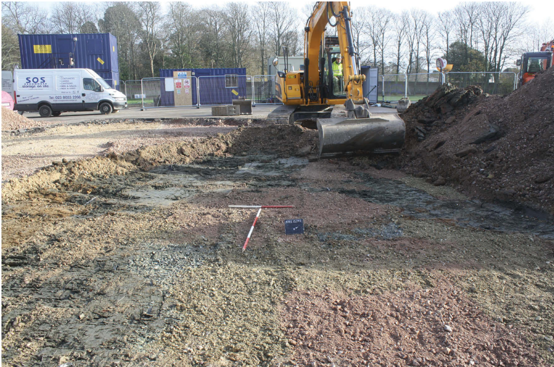
Plate 1. Overburden stripping in progress with some brickearth exposed (grey), looking east, Scales: 2m and 1m.
