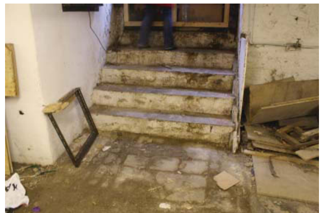
Plate 16. Interior, room A, stone slabs next to entrance steps, looking south east.
