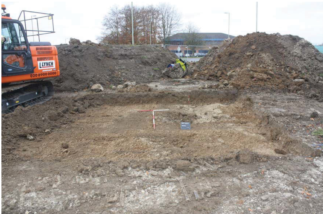
Plate 1. Antennae base area after topsoil strip, looking west, Scales: 2m and 1m.
