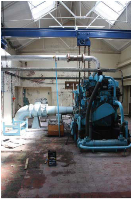
Plate 17. Pumping equipment in room 9, looking East.
