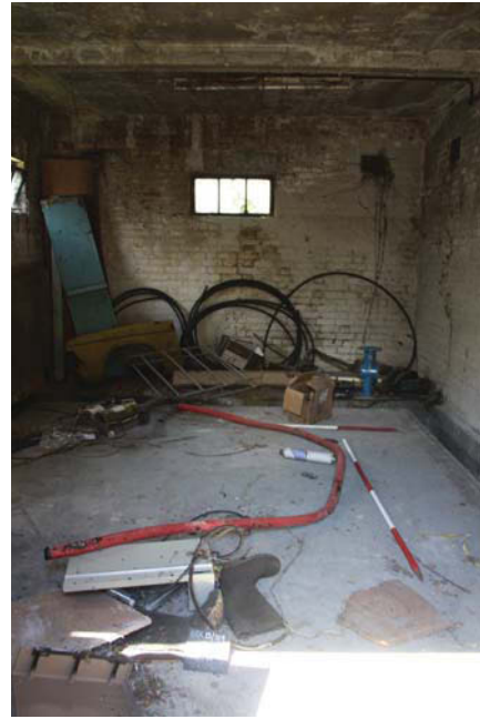
Plate 22. Internal view of substation, looking North, Scales: 2m and 1m.
