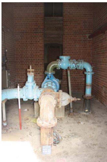
Plate 11. Pumping equipment in room 5, looking North, Scale: 1m.
