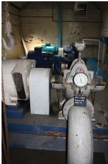
Plate 15. Pumping equipment in room 8, looking North.
