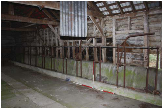
Plate 7. Interior, Unit A, concrete troughs, looking north west, Scales: 2m and 1m.
