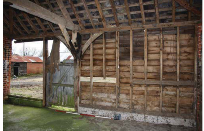
Plate 26. Interior, south facing interior wall of Unit C, Scales: 2m and 1m.
