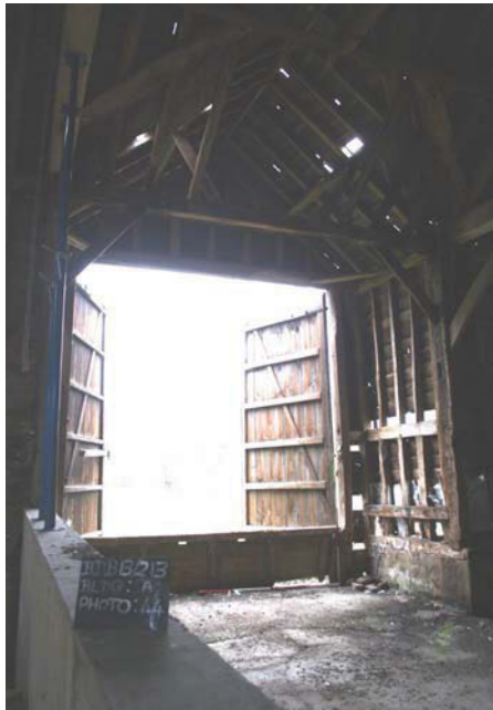
Plate 13. Interior, Unit A, interior door Unit A, looking north east, Scales: 2m and 1m.
