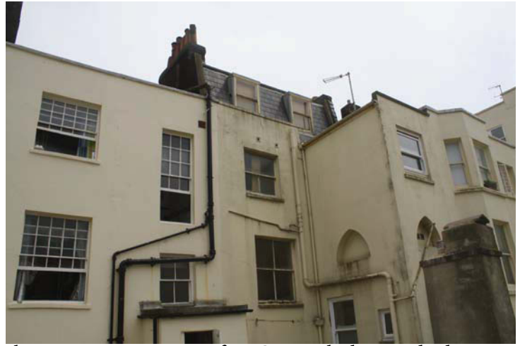
Plate 22. Exterior, rear of 33 Oriental Place and adjacent properties to south, looking SE from roof terrace
