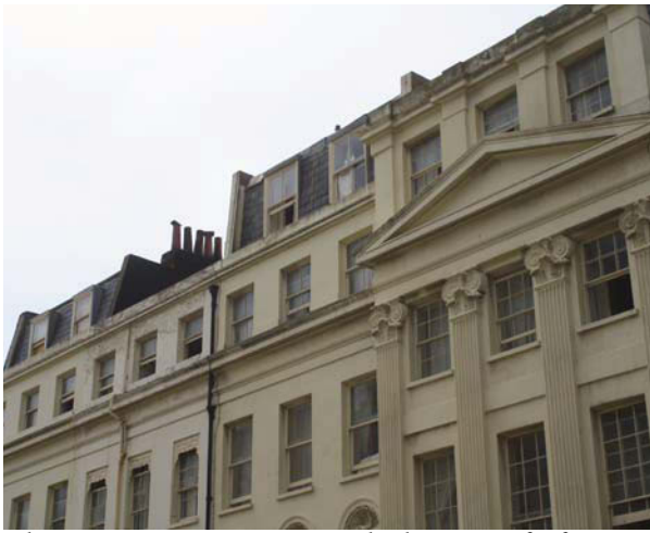
Plate 25. Exterior, Oriental Place, roof of 33 Oriental Place and adjacent properties, looking SW
