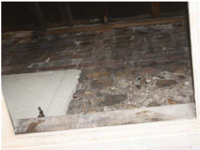
Plate 7. Interior, southern loft, south wall looking up from shower room C, looking SSW
