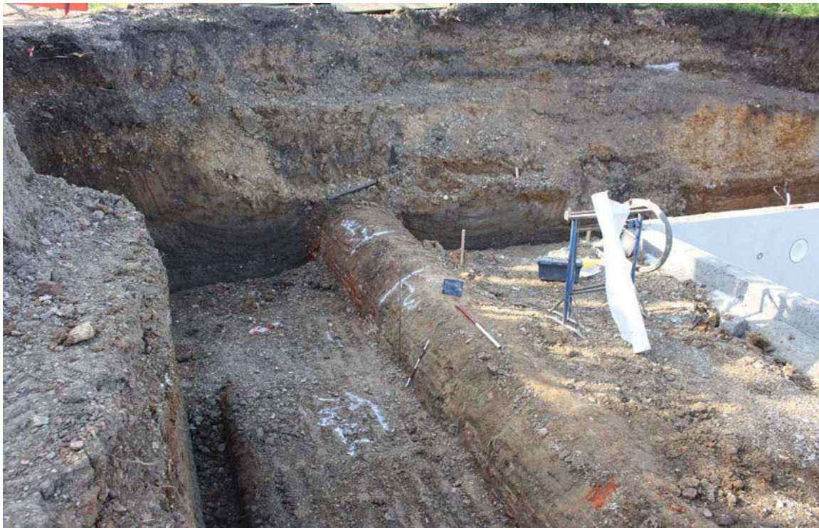
Plate 9. Tunnel (61) showing cut 4 in section, looking south across reduced area for pool and its retaining wall. Scales:1m
