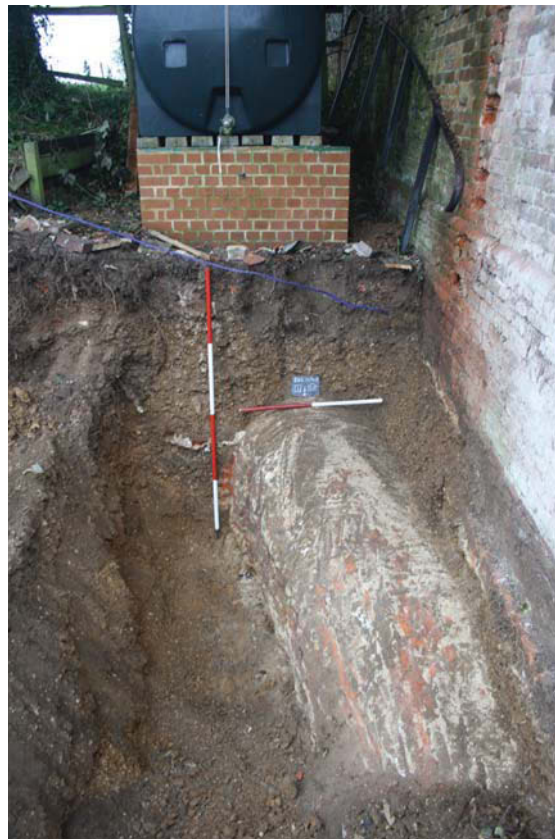
Plate 2. View of tunnel cut (1) before opening, looking south, Scales: 2m and 1m
