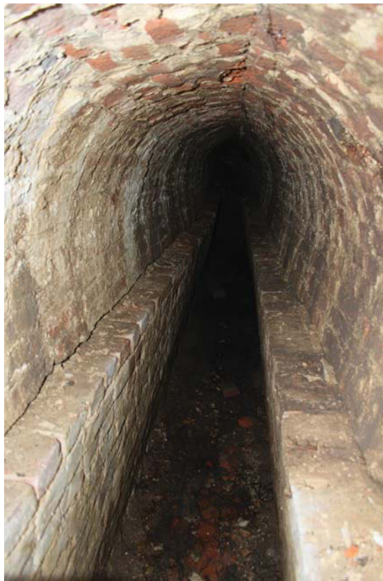
Plate 4 General view of tunnel, looking north from entry point showing subsidence with blockage beyond, Scales: 2m and 1m
