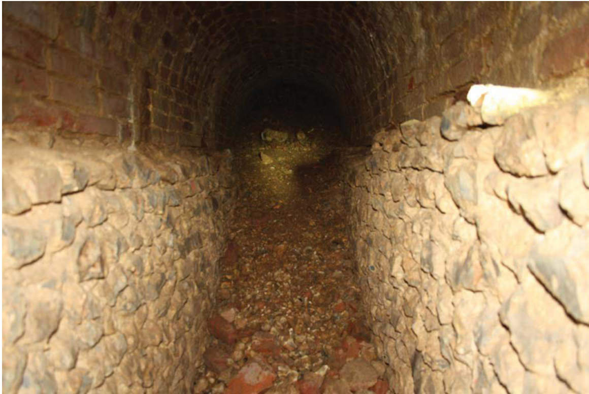
Plate 5. General view of tunnel blockage at south end, looking south
