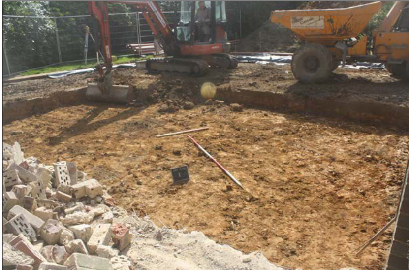
Plate 1. Eastern area of reduction under slab, looking south, Scales: 2m and 1m.
