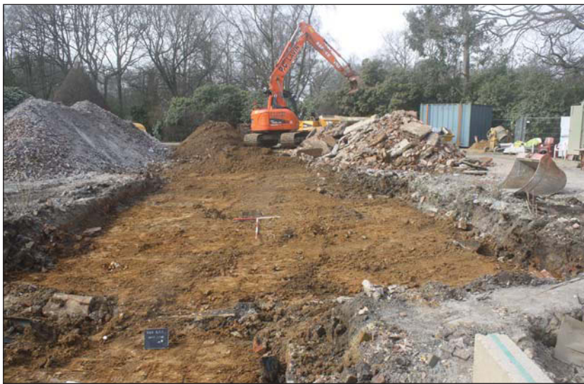
Plate 2. Reduction on site of previous building, looking north west, Scales: 2m and 1m.
