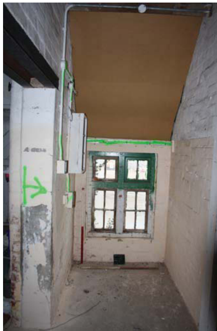
Plate 11. Window in room 5, looking southeast, Scales: 2 x 1m..
