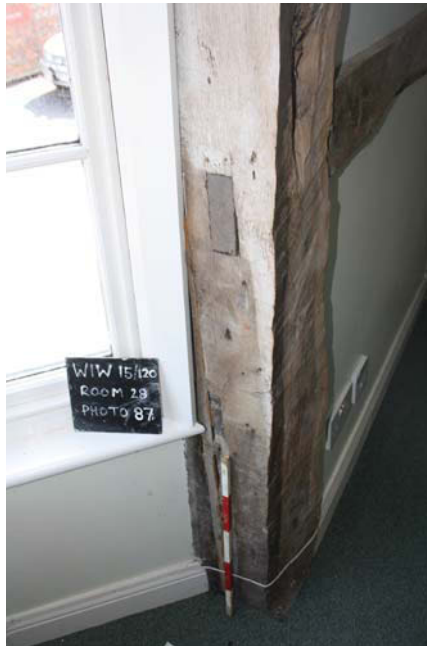
Plate 25. Room 28, detail of cut rail in window area , looking east. Scale 0.5m.
