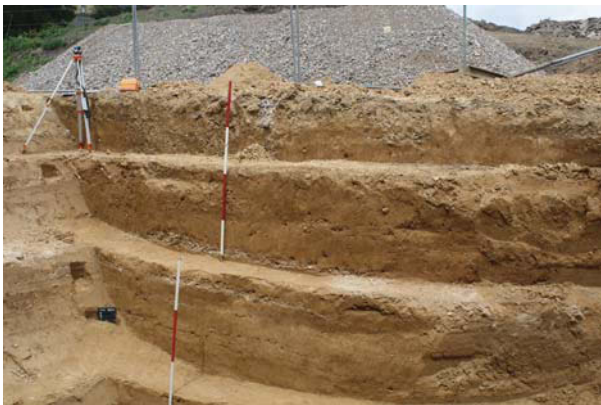
Plate 3, View of upper test pit after excavation, looking north west, Scales: 2m
