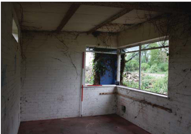
Plate 7. View to windows within structure A, looking southwest. Scales: 2m and 1m.
