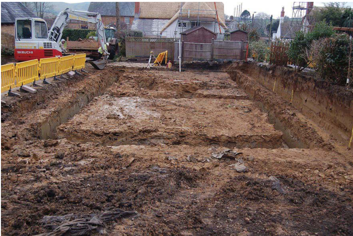
Plate 2. The site after excavation of the foundation trenches, looking south (2m scale)
