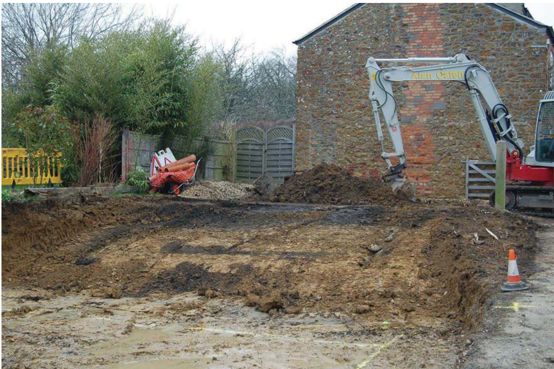
Plate 4. Modern disturbance and land drain at the north end of the site, looking north-west (no scale)
