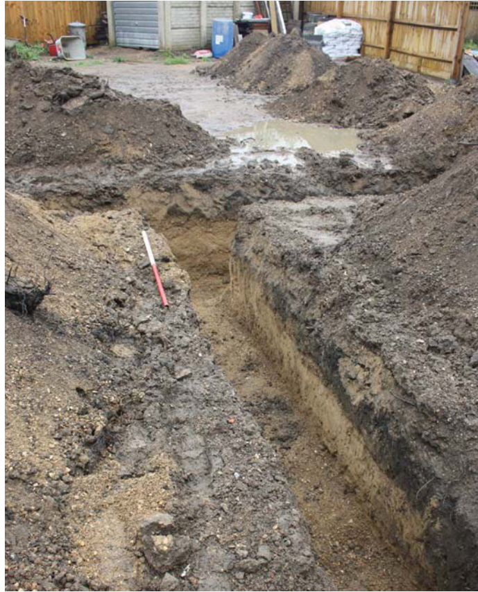
Plate 1. Footing at close to location of Trench 2 , looking north north east, Scales: 1m.
