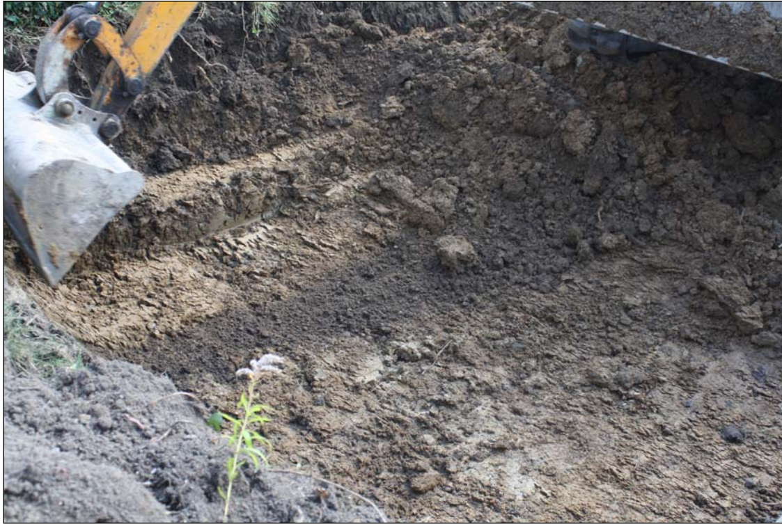
Plate 1. View of site during stripping: the dark stripe is merely loose soil, not a feature
