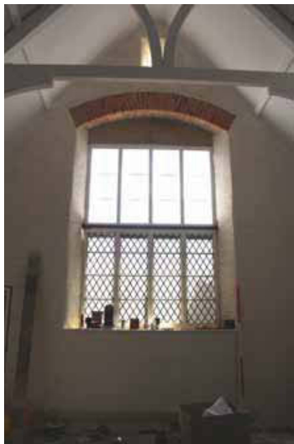
Plate 13. View to window in east gable end, looking East, Scales: 2m and 1m.
