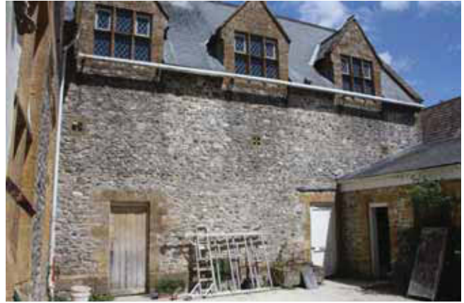
Plate 6. South elevation of north range (within yard area), looking North, Scales: 2m and 1m.
