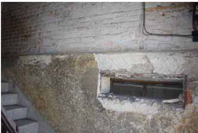
Plate 31. TBlocked window detail?, looking West.
