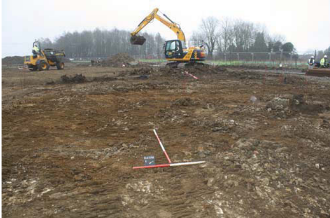
Plate 1. General site conditions during stripping, Block A, looking south-east, Scales: 2m and 1m.
