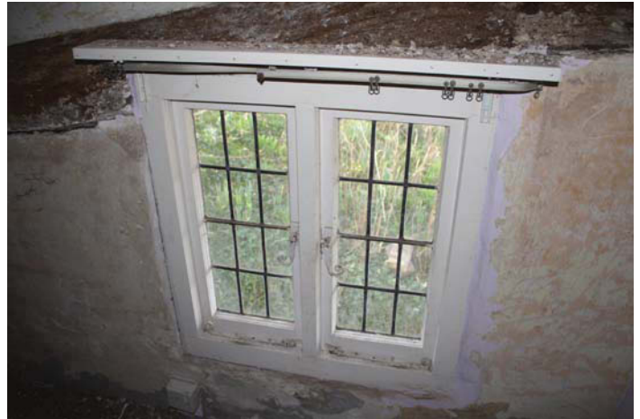
Plate 10. Bedroom C during building work, detail of window in S wall, looking SSE.
