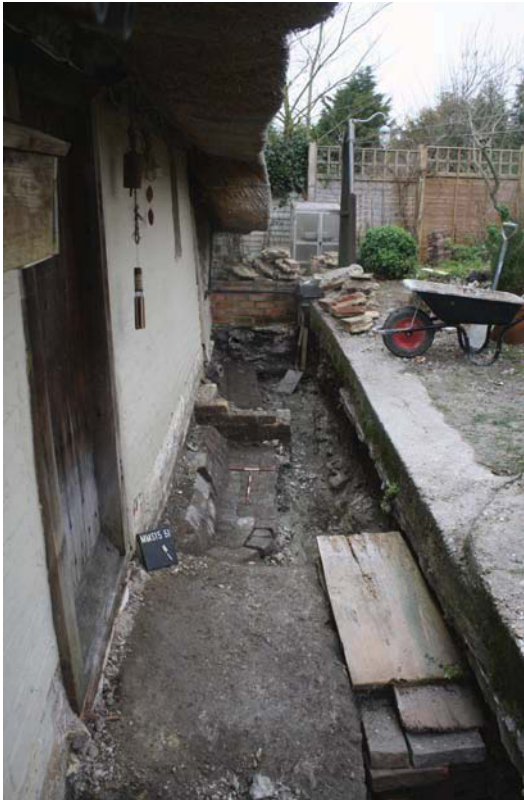
Plate 1. Drain 51 and trench around east side of house, looking north-east; Scales 0.5m and 0.3m.
