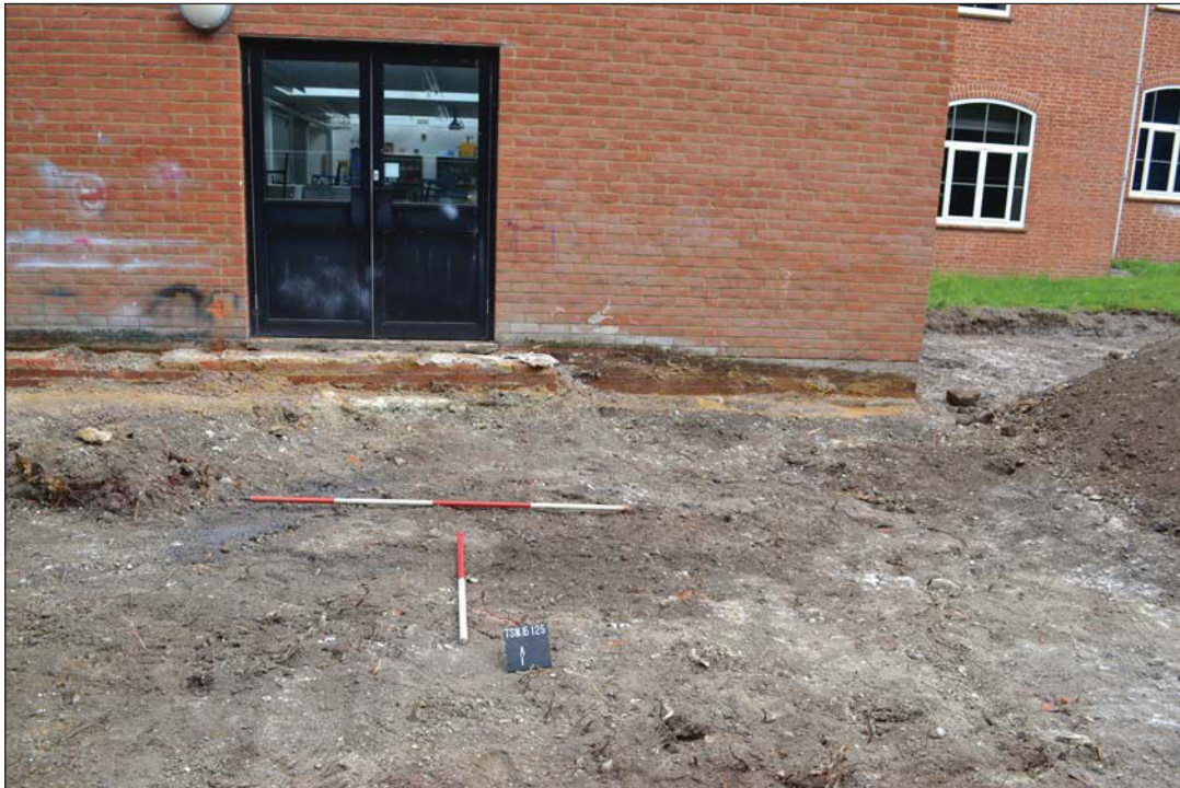
Plate 1. Initial ground reduction and location of site looking north, Scales: 2m and 1m.
