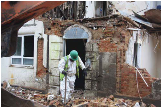
Plate 13. Scar either side of front door, looking North north-east.
