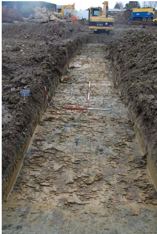
Plate 2. Trench 6, looking south south west, Scales: horizontal 2m and 1m, vertical 0.5m.
