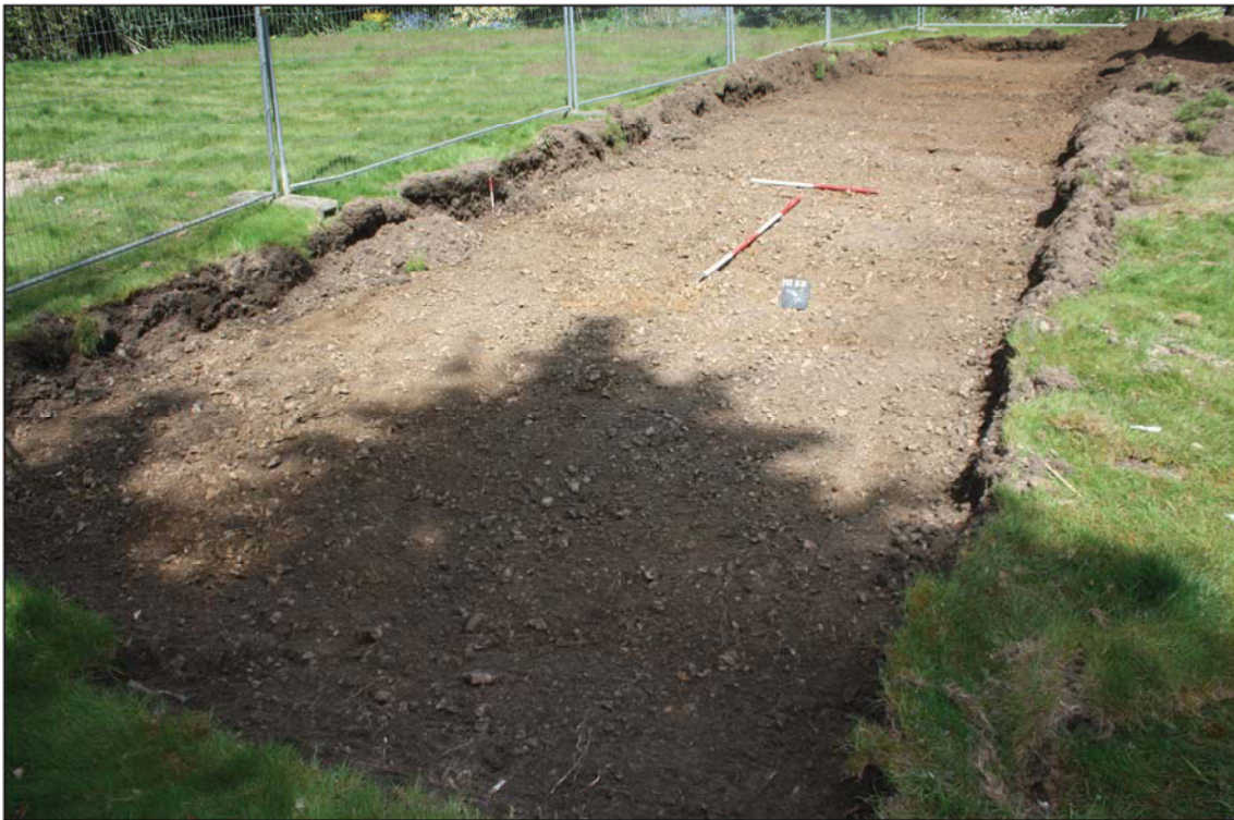
Plate 1. Strip for soakaway, looking north east, Scales: horizontal 2m and 1m, vertical 0.3m.
