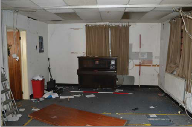
Plate 9. Interior, Counting House ground floor, room 4, looking north north west, Scales: 2m.
