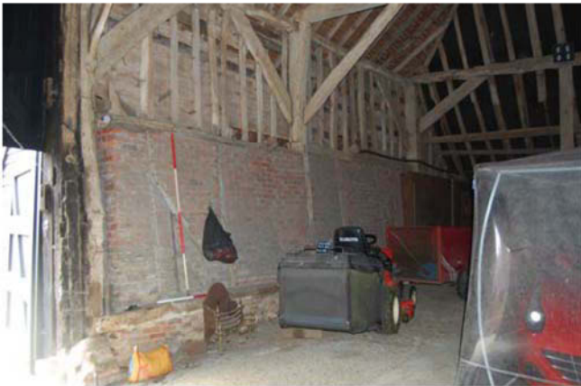
Plate 5. Northwest barn south wall detail (lower), looking south-southeast, Scales: 2m and 1m.
