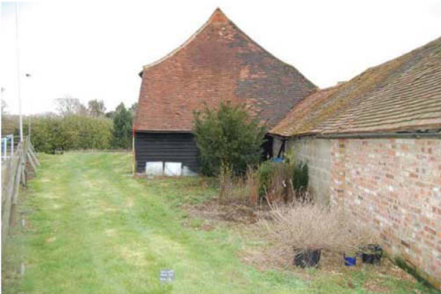
Plate 11. West wall of NW barn and rear of cart-shed, looking east, Scales: 2m and 1m..
