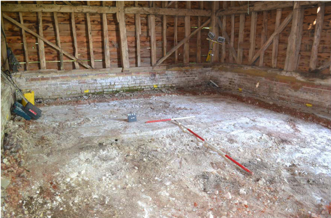
Plate 1. Eastern side of barn interior after ground reduction, looking south east, Scales: 2m and 1m.
