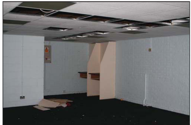
Plate 30. Q4, snooker room showing blocked windows, looking east-southeast.
