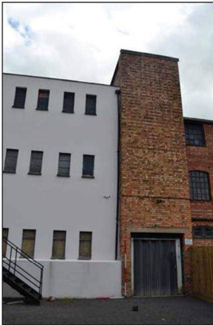
Plate 7. Exterior, original building, front elevation, centre, looking southeast, Scales: 2m and 1m.
