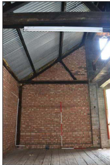
Plate 24. Room 23, view to gable end of northwest extension, looking northeast Scales: 2m and 1m.
