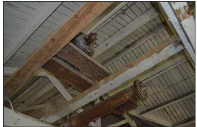
Plate 40. Room 26, Motor and wheel detail, looking south.
