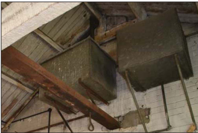
Plate 35. Room 25, Tanks within roofspace detail, looking northwest.
