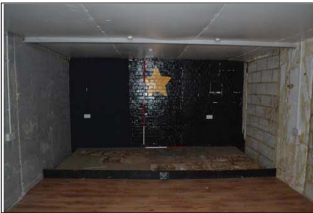
Plate 19. Room 12, general view showing blockwork infill, looking southeast, Scales: 2m and 1m.
