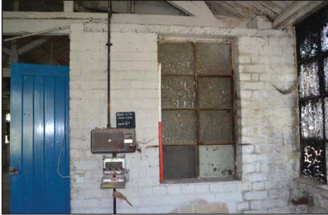
Plate 37. Room 26, Stairwell window and motor controls, looking southwest, Scales: 1m.
