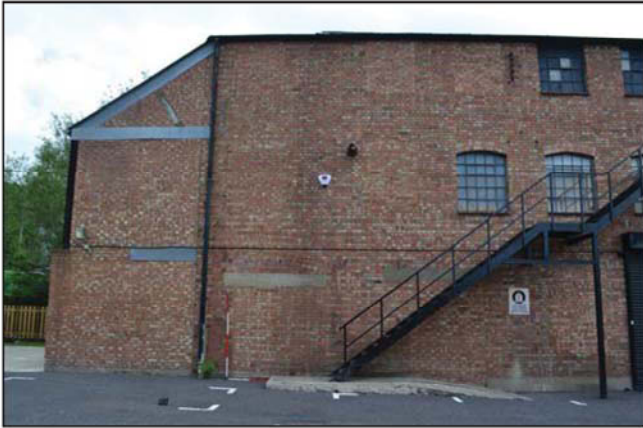
Plate 5. Exterior, original building, front elevation, north-west end, looking southeast, Scales: 2m and 1m.
