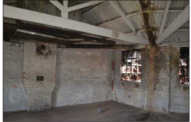
Plate 38. Room 26, Blocked door in gable end and tank in roofspace, looking north, Scales: 2m and 1m.
