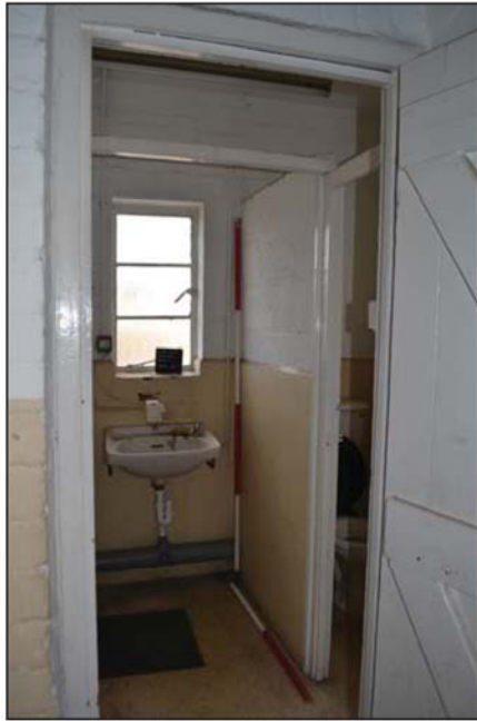
Plate 29. Room 7, View to toilet and sink, looking south, Scales: 2m and 1m.
