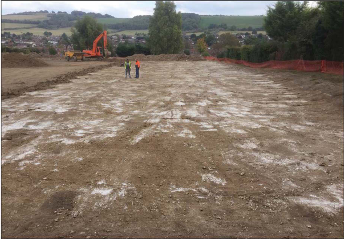
Plate 1. General view showing southern part of site following initial topsoil removal, looking ENE.
