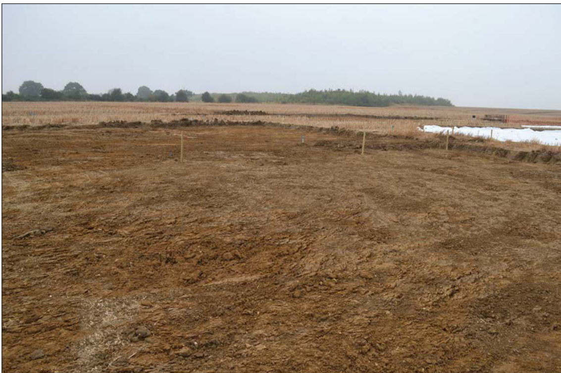
Plate 4. Topsoil strip over overflow car park, looking south west, Scales: 2m and 1m.
