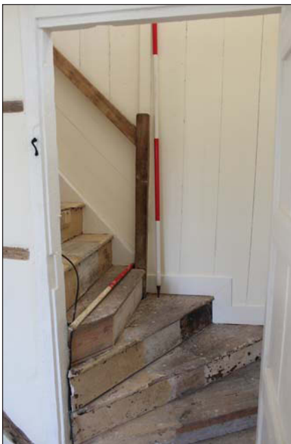
Plate 13. Bottom of the stairs and plank wall detail, looking north east, Scales: 2m and 1m.
