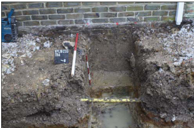
Plate 3. Footing trench showing footings of existing house, looking West south west. Scales: 1m and 0.5m.
