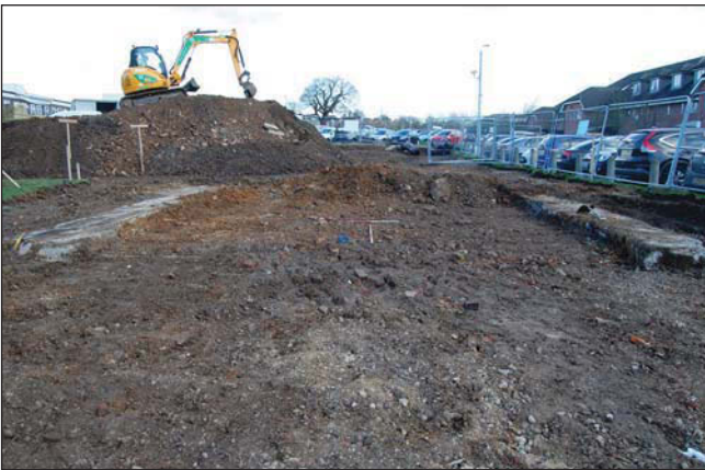
Plate 3. Area A, concrete footings of building, looking west, Scales: 2m and 1m.
