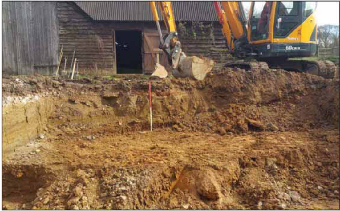
Plate 1. Area under excavation, uncovering upper layers, looking east north east, Scale: 1m.
