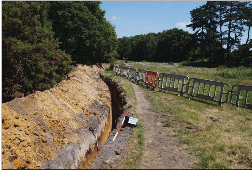
Plate 1. General view along the western pipe trench area, looking east, Scales: 2m and 1m.
