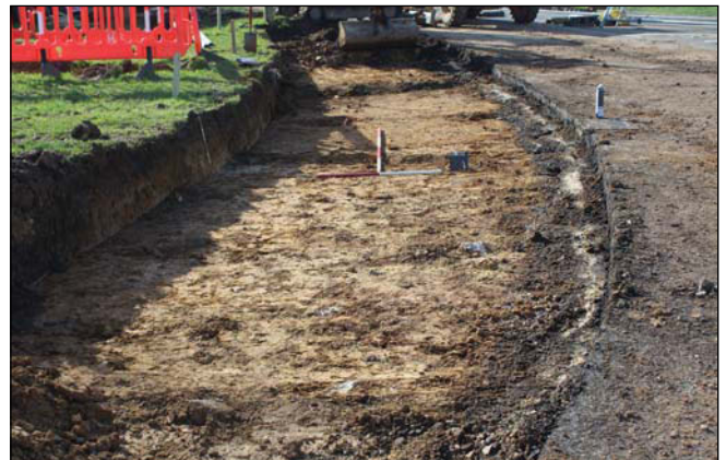
Plate 7. General view of Mitigation Area B, looking South. Scales: 2m and 1m.
