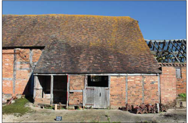
Plate 30. Exterior, Courtyard, north barn, south elevation, looking north, Scales: 2m and 1m.
