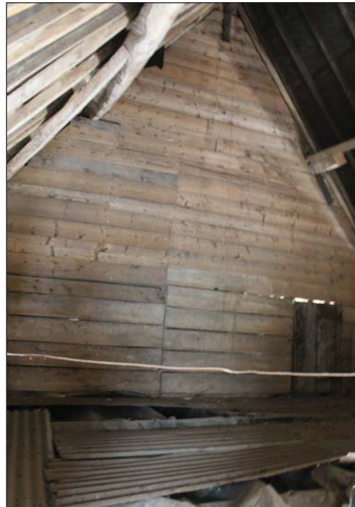
Plate 22. Interior, north barn, from Bay 3 stairs looking at Truss 3, looking south east.
