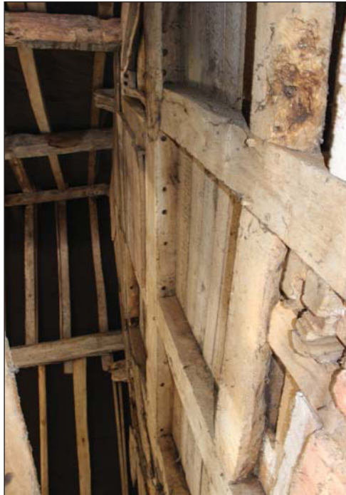
Plate 9. Interior, north barn, Bay 5, roof space looking at Bay post and truss (4).
