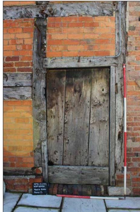
Plate 14. Exterior, north barn, western gable, doorway detail, looking east, Scales: 2m and 1m.
