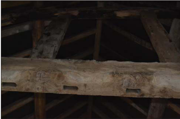
Plate 29. Interior, north barn, roof detail, removed post slots on underside of roof truss.
