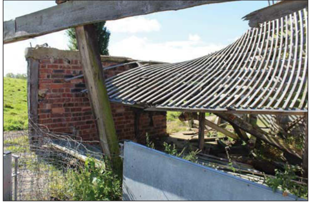
Plate 46. Exterior, south barn, collapsed roof.
