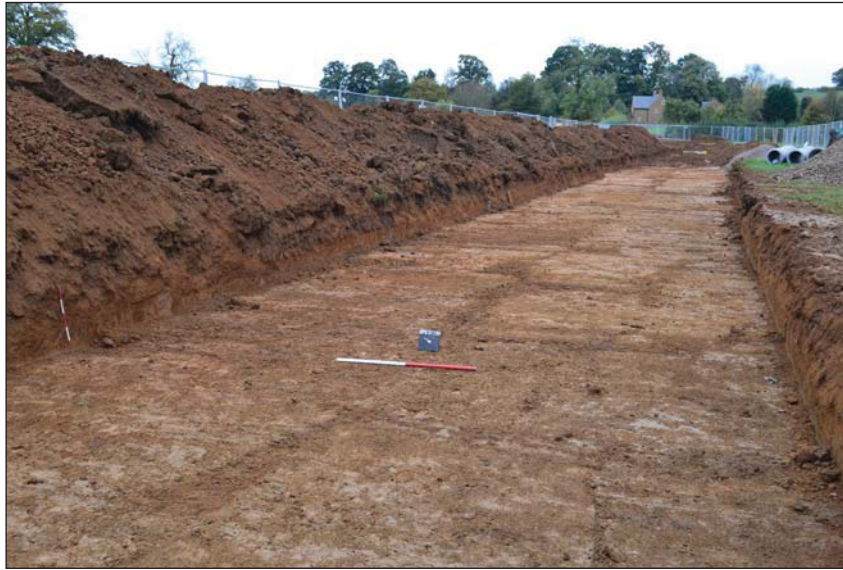
Plate 3. Route of pipeline stripped, looking to SW, Scales: horizontal 1m, vertical 0.5m.
