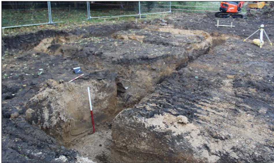
Plate 3. Western side of new footings, looking north west, Scales: 1m and 0.5m.
